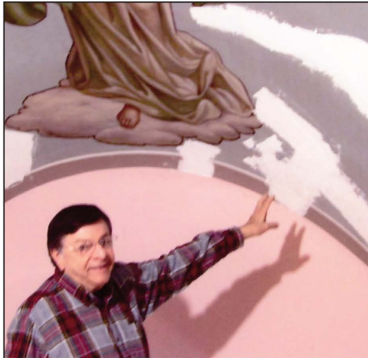
James J. Pecorelli, senior project manager for Baker Liturgical Art, shows one of many locations in the ceiling needing reinforcement. Wall and ceiling portions had actually become flexible, and if not attended to soon, large chunks would have started to tear away, he said
