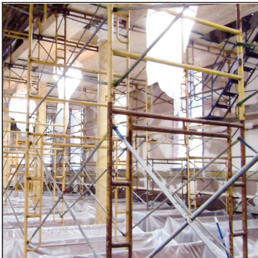
Scaffolding lines the interior of St. Stephen's Church in Croghan, supporting workers three and four levels above. Parishioners who are currently worshipping in the church basement are expecting to be seeing a completed renovation by Memorial Day.
