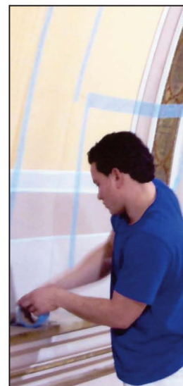
Carlos Jaramilla, Queens, tends to resin work along the walls beneath the ceiling.
